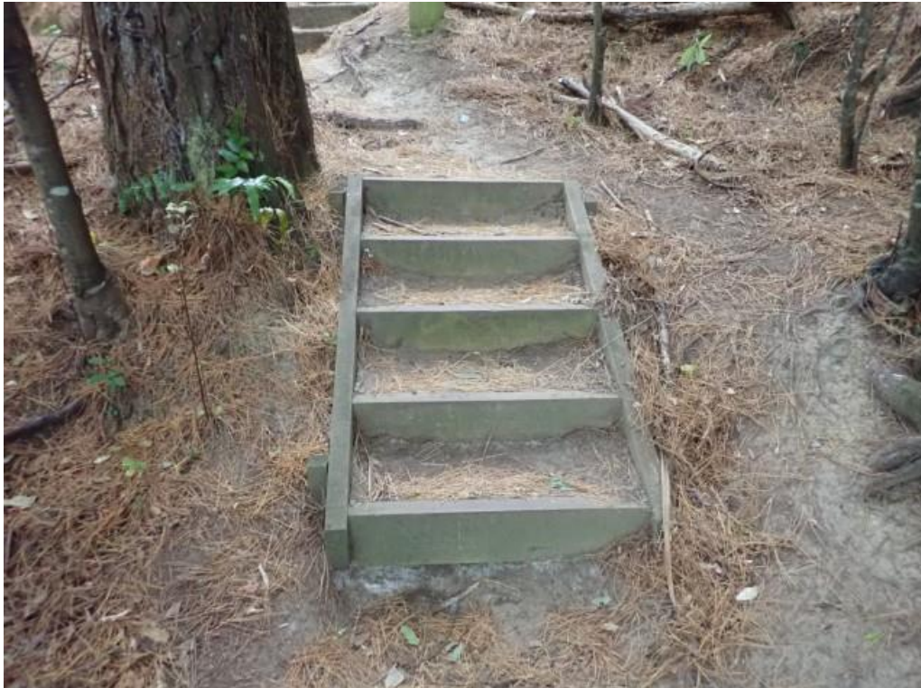
Photo 9: 5 steps just below unmarked bollard
