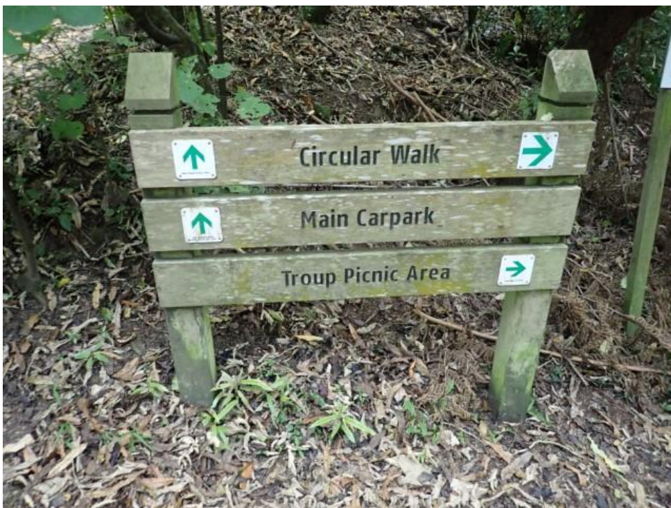
Photo 28: Wayfinding sign Comment: Maintenance required. Recommendation: Sand/plane the front surface only and reinstate appropriate arrows. The signs will look like new. When due for replacement, suggest changing 'Main Carpark' to 'Wilton Rd Carpark'.
