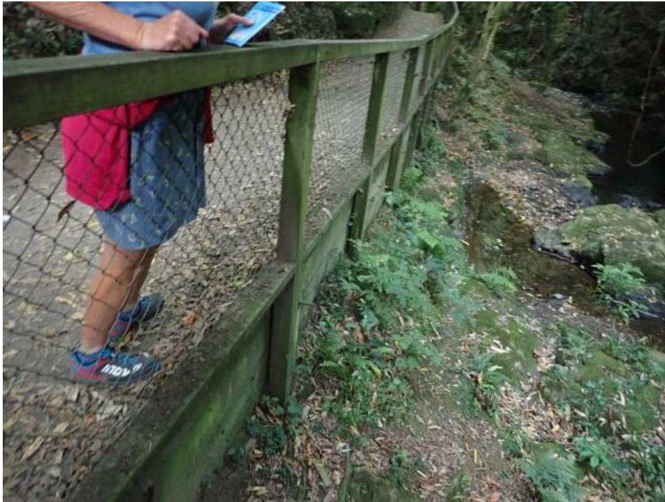
Photo 27: Retaining wall on Kaiwharawhara Track Comment: Fencing required because of drop to stream. Recommendation: None.
