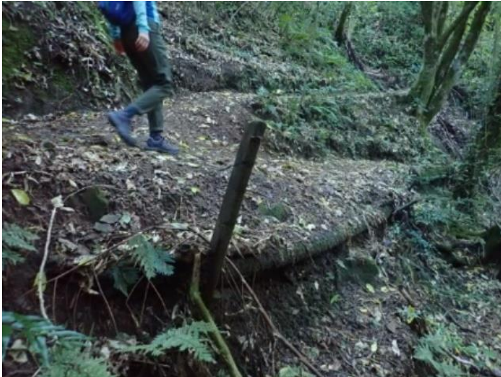
Photo 5: Failing retaining wall
