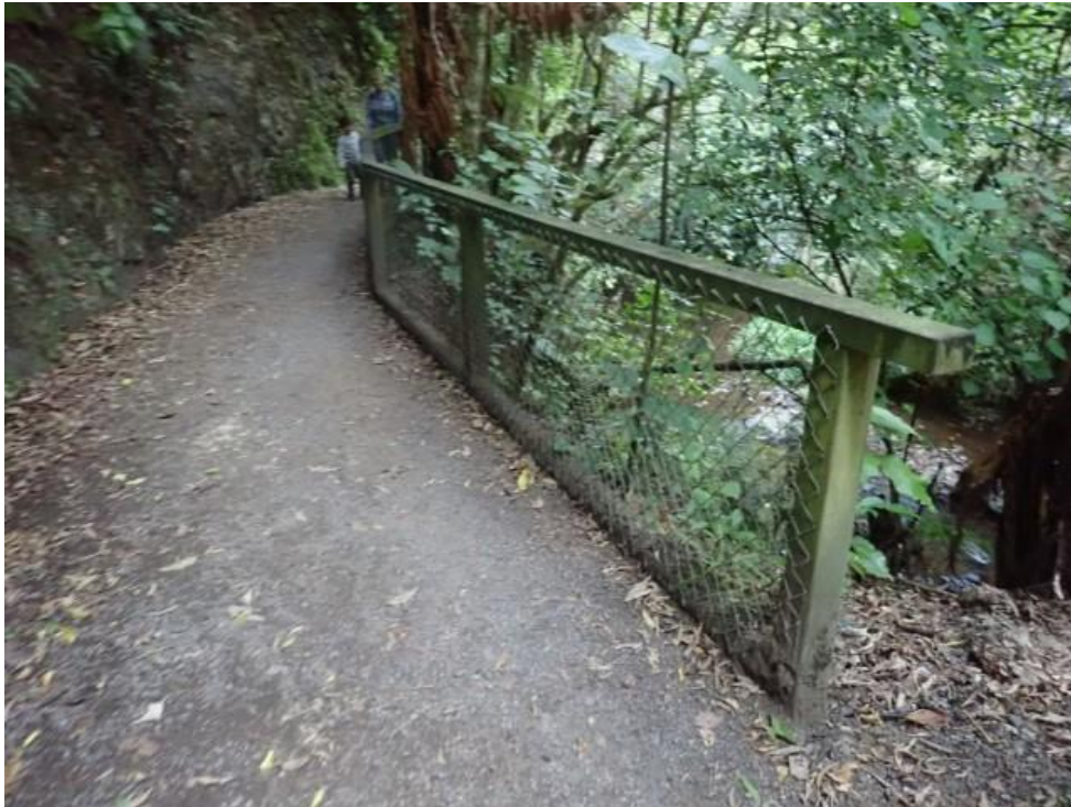
Photo 4: Barrier to stream
