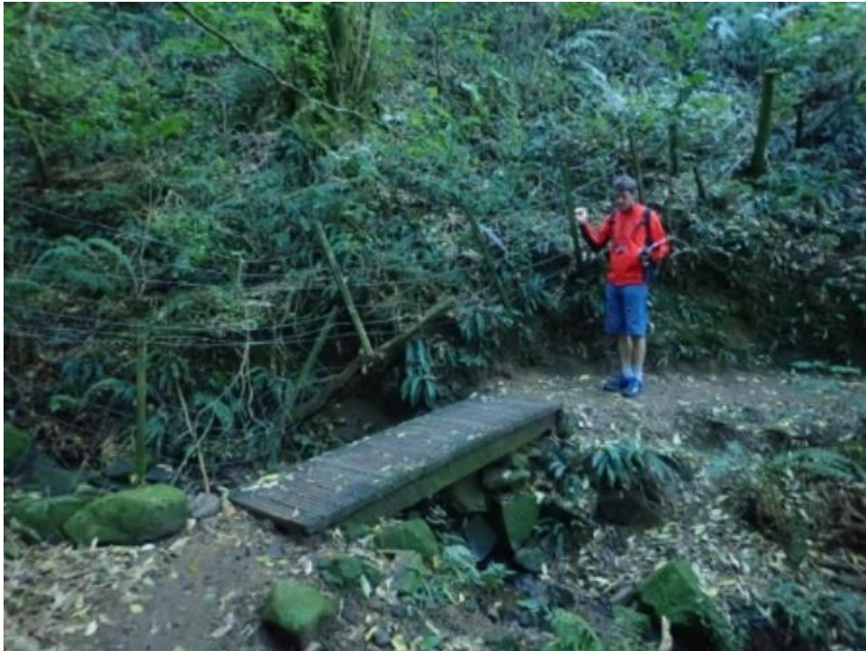
Photo 11: Boardwalk (3m by 0.7m) and old fence hanging over the track
