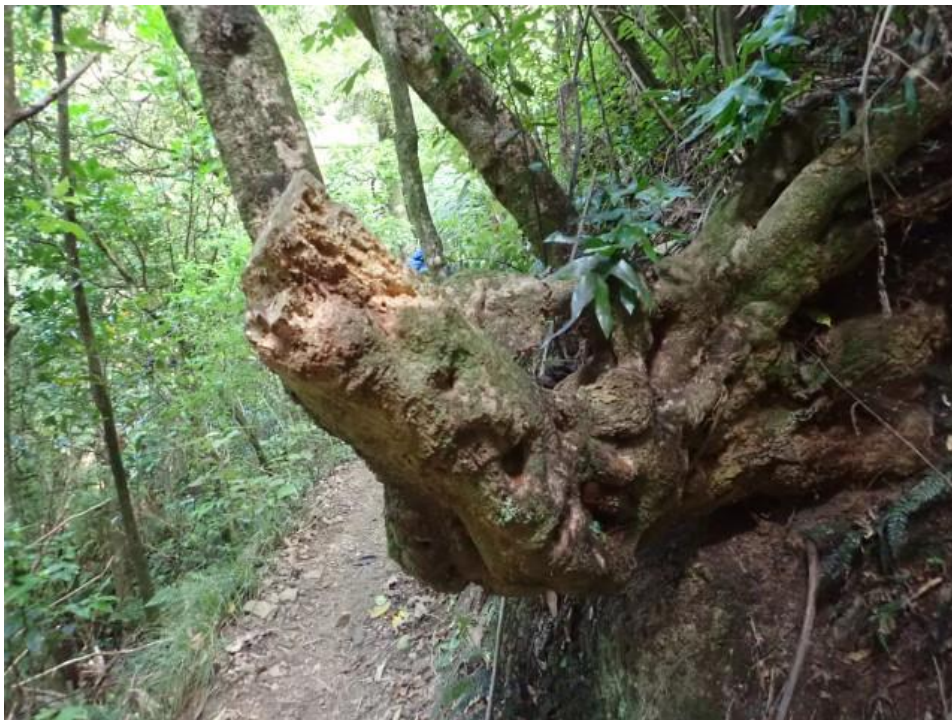
Photo 42: Rotting stump Comment: This old mahoe stump encroaches on the track corridor, pushing users towards the outside edge. Recommendation: Cut flush to the track bank.
