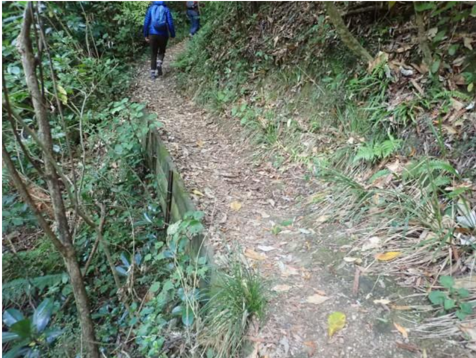
Photo 41: 7-metre-long retaining wall, up to 0.8 metres high; five waratahs Comment: The waratahs look in OK condition but should be replaced within 10 years. Recommendation: Schedule replacement of waratahs.
