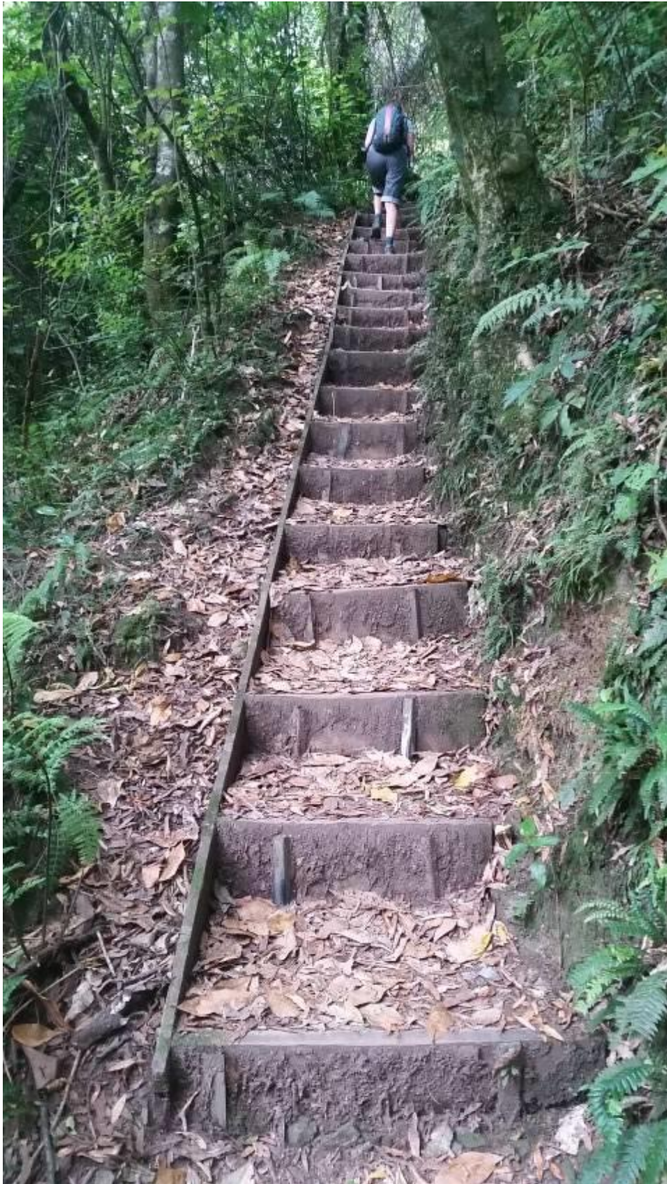
Photo 28: 18 of the 48 steps. Some are now up to 400mm high because the soil at the bottom of the boards has compacted/eroded.
